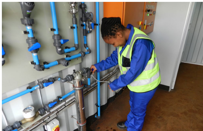
Regular checks guarantee the drinking quality. ©Virtual Consulting Engineers VCE, Mark Woods
