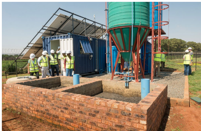
Demonstrator in South Africa: overall view including the solar panels supplying the electrical power needed. ©Fraunhofer IST, Jan Gäbler
