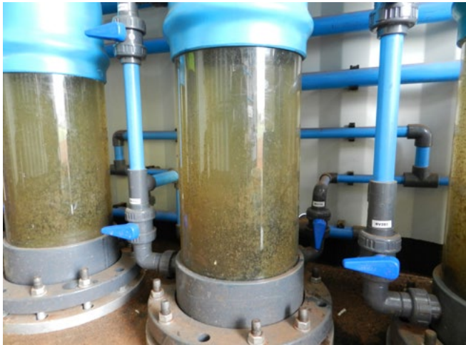
Coagulation and flocculation columns for purifying the river water. © Fraunhofer IST
